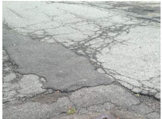
A14 _Gaston Street parking lot - mill and repave, restripe, proper ADA signs and layout
