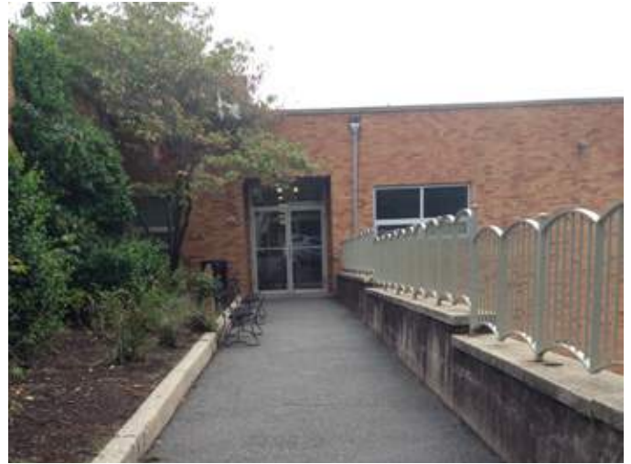
A8 _Trim trees overhanging the roof
