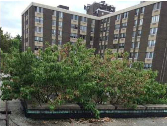
A9 _Trim trees overhanging the roof
