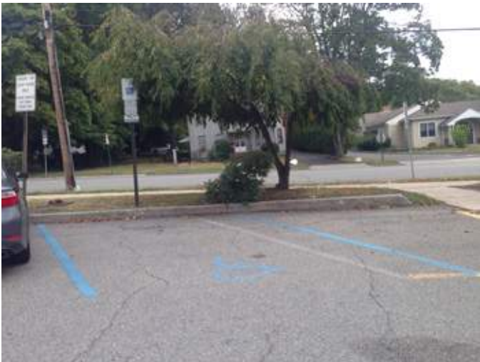
A13 _Gaston Street parking lot - mill and repave, restripe, proper ADA signs and layout
