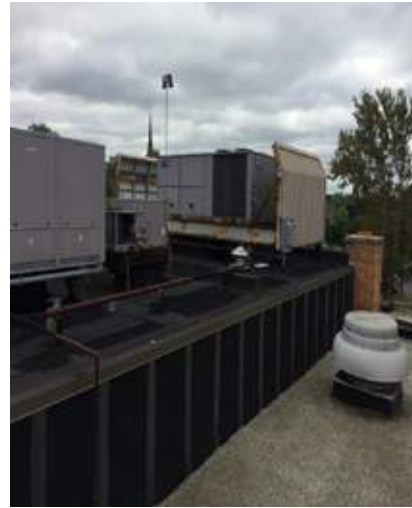
E2_RTU's on Roof
