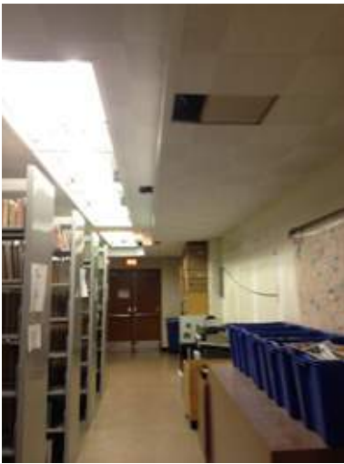
A25 _Paint walls and replace wall base at lower level storage/stack area
