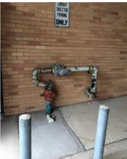
E5_Gas Service and Meter on Outside
