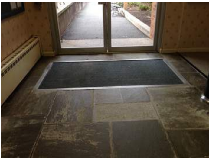
A33 _Tripping hazard and ADA issue at entrance walk-off mat pockets-replace mats
